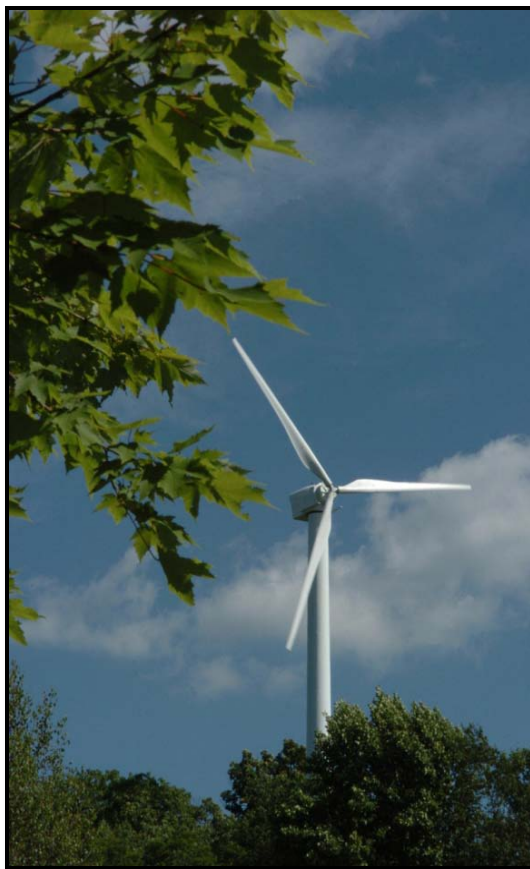
Figure 10: A Northern Power Systems North Wind 100 Wind turbine generator located on the campus of Appalachian State University. Photo courtesy of Appalachian State University
