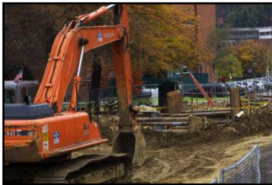
Figure 2: Construction along River Street to improve the steam loop. Photo by Jordan Paris
