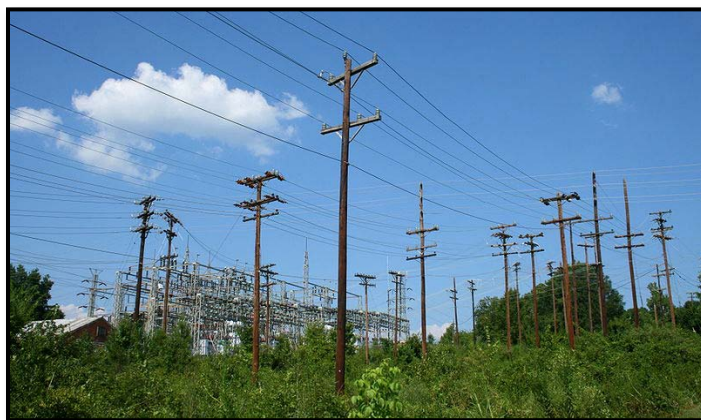
Figure 6: Utility transmission lines
